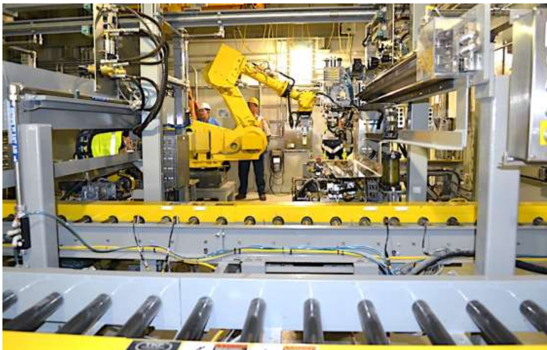
Figura 104. Transportuesi horizontal, Pueblo Chemical Agent-Destruction Pilot Plant
